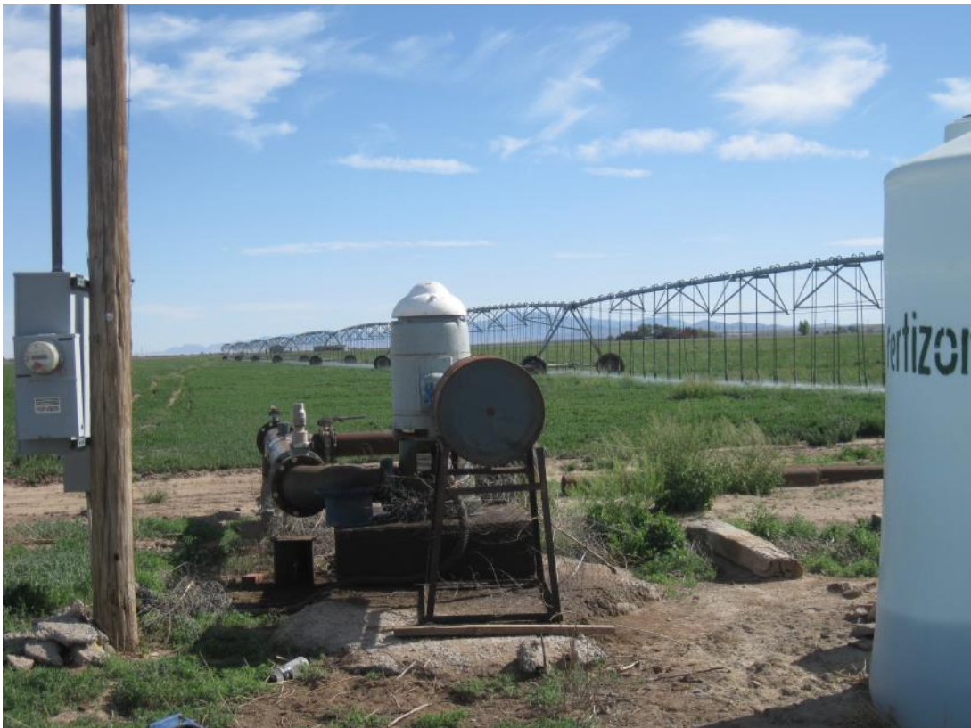
Well 1, approx. 600' deep, 16" casing, 75 hp, 700 gpm
